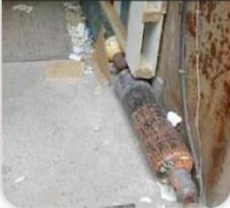
COMPRESSED GAS UNSAFE STORAGE
