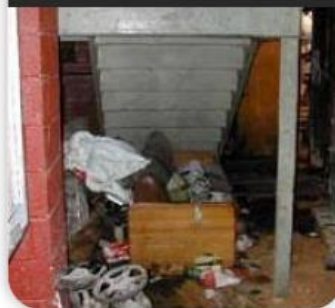
STORAGE IN STAIRWELL
