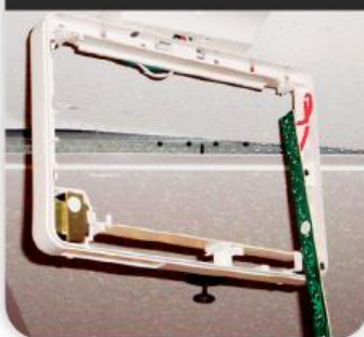
EXIT SIGN INOPERABLE
